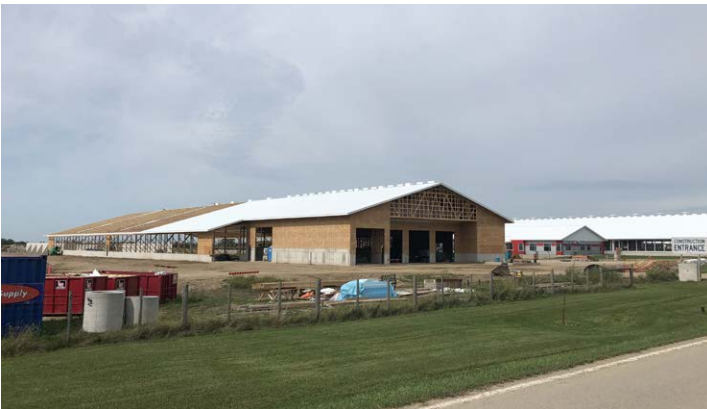
The new cow barn and some of the renovated pastures at the University of Guelph's research farm near Elora, ON are now in use, and work is nearly done on the construction of the new feedlot barn.
